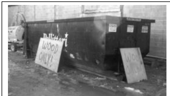
Figure 9. Findorff workers created these spray-painted plywood signs to label dumpsters after they were moved around to re-open Mifflin Street. May 2003.
