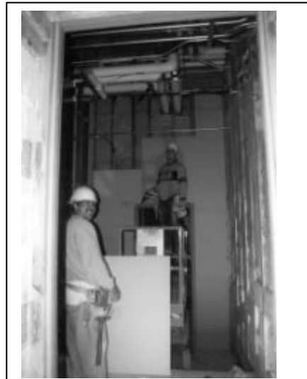
Figure 8. When visiting the construction site, we talked to subcontractors, and to Findorff workers (such as these workers installing drywall) about recycling. May 2003.
